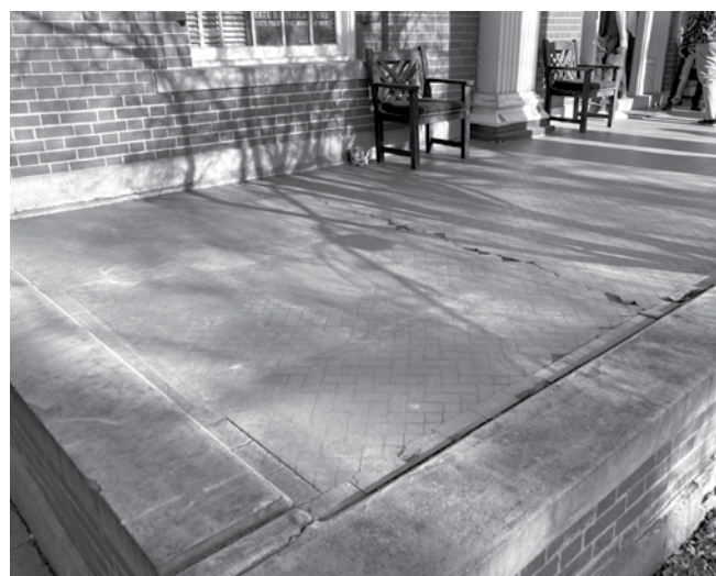
Both the herringbone pattern and the historic terra cotta tile have been restored at the Bennett-Field House. Photo: Mike Owen
